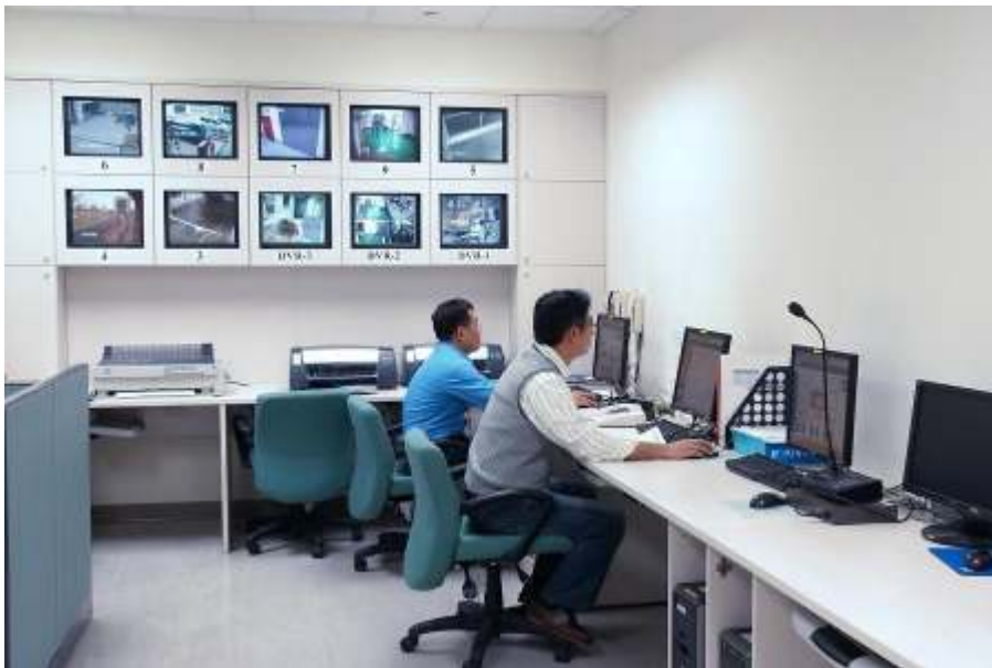
Central Control Room
