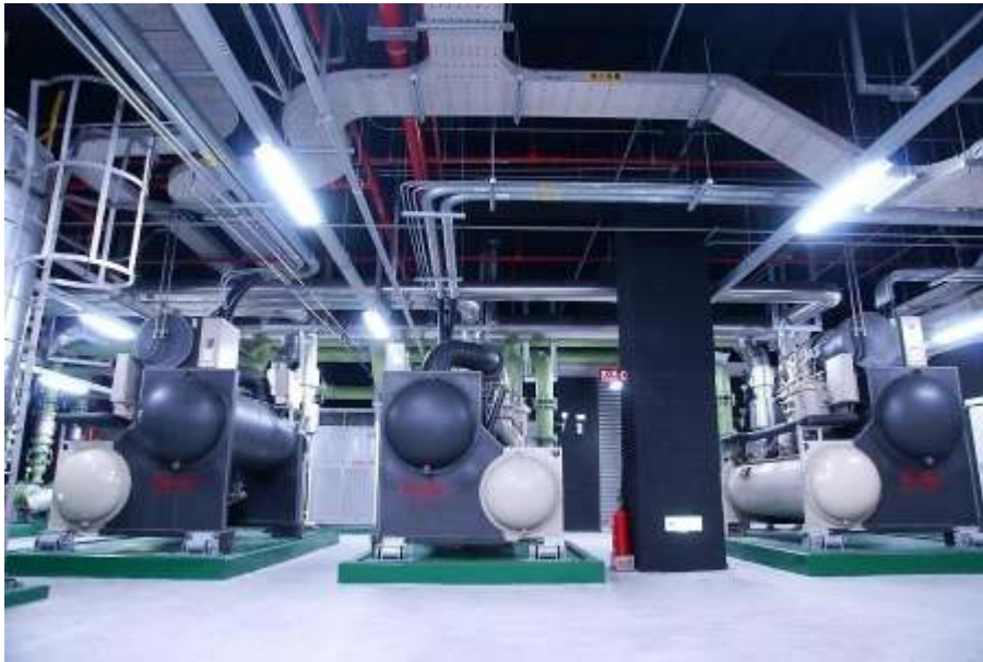
Yankee Center, NHRI HVAC system 空調冰水主機
